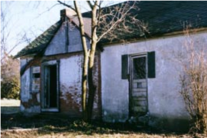
Fig. 5. The north side of the house still shows plenty of evidence of the removed kitchen ell.
