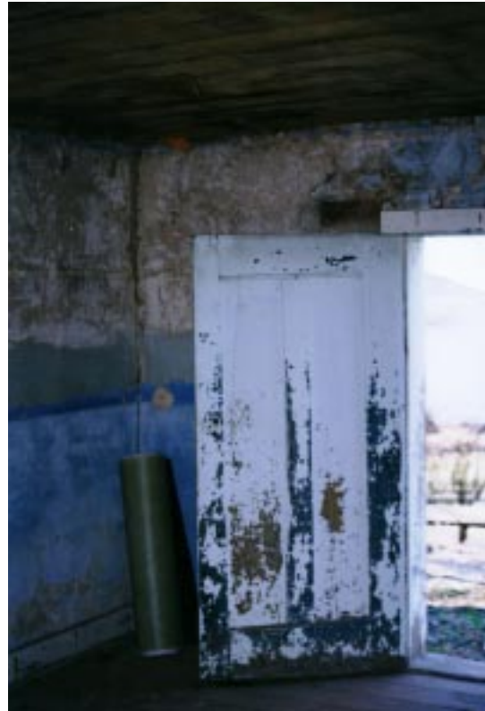
Fig. 4. This blue and tan two-panel door probably is original to the east room addition of the house.
