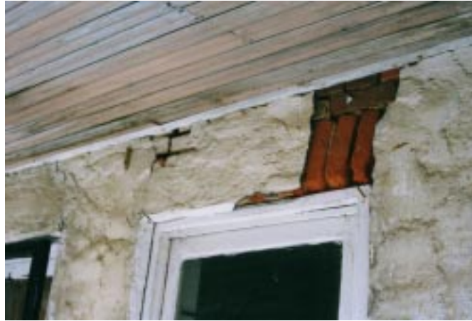
Fig. 9. Fallen stucco reveals a decorative flat brick arch over the south window in the east room addition.
