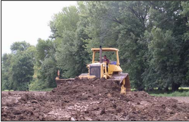
Photo of earthwork being done to construct one of the berms on a 125 acre impoundment.
