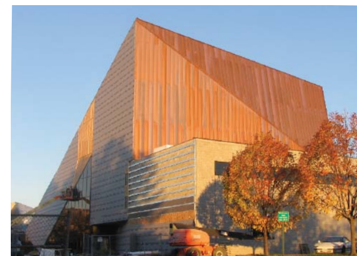
Construction continues on the Doudna Fine Arts Center with completion anticipated in Spring 2008.
